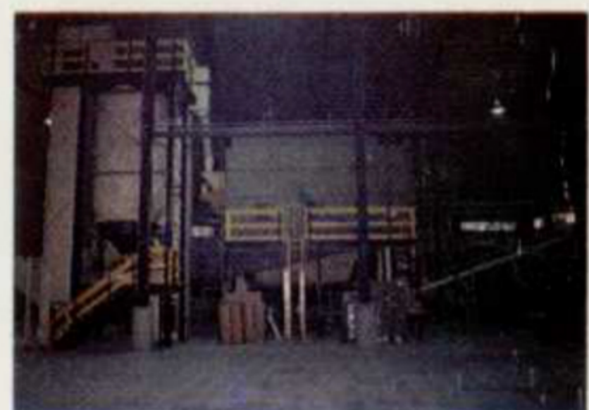
The LESCO facility in Martins Ferry, Ohio is the largest sulfur-coating plant in the world.
