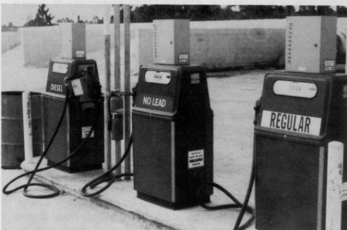
Fueling Island at Martin Downs with approved fire extinguisher.
