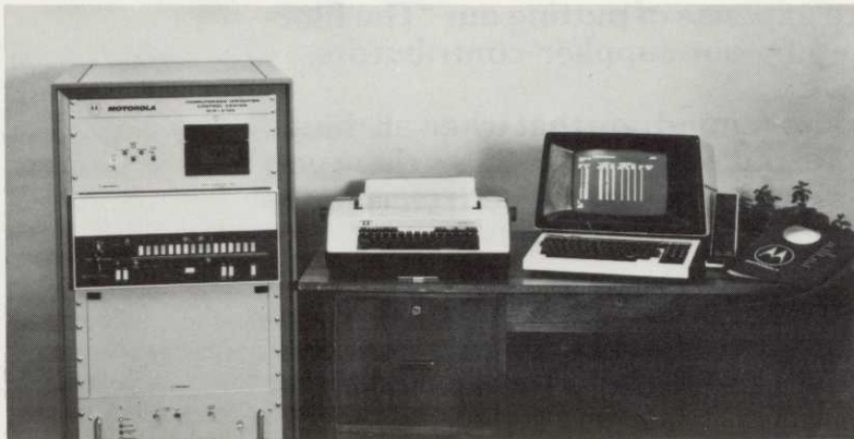
MIR-2100 CENTRAL STATION, City of Los Angeles Encino Golf Course (Installed by California Engineering, Sylmoor, CA)
