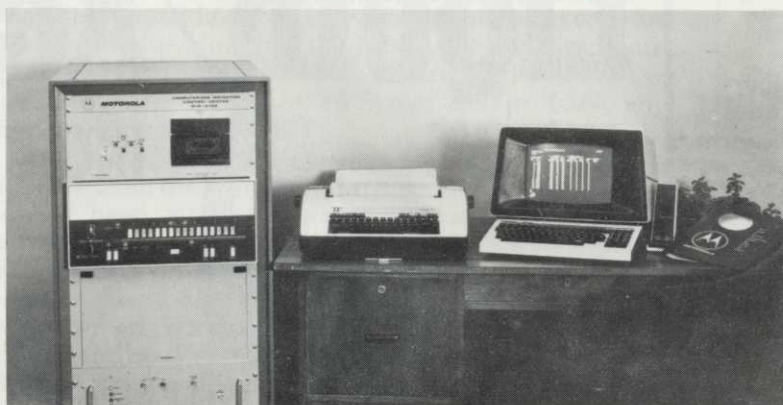
MIR-2100 CENTRAL STATION, City of Los Angeles Encino Golf Course (Installed by California Engineering, Sylmar, CA)
