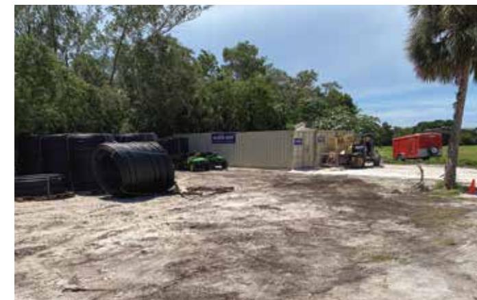
The staging area for Liebold Irrigation at Longboat Key Club is proof that partially District-funded work is underway.
