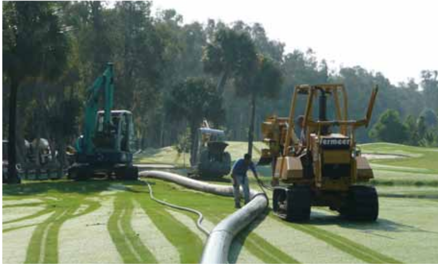
Recent Estero irrigation upgrades improved turf quality and helped reduce costs. Photo by Shelly Foy.
