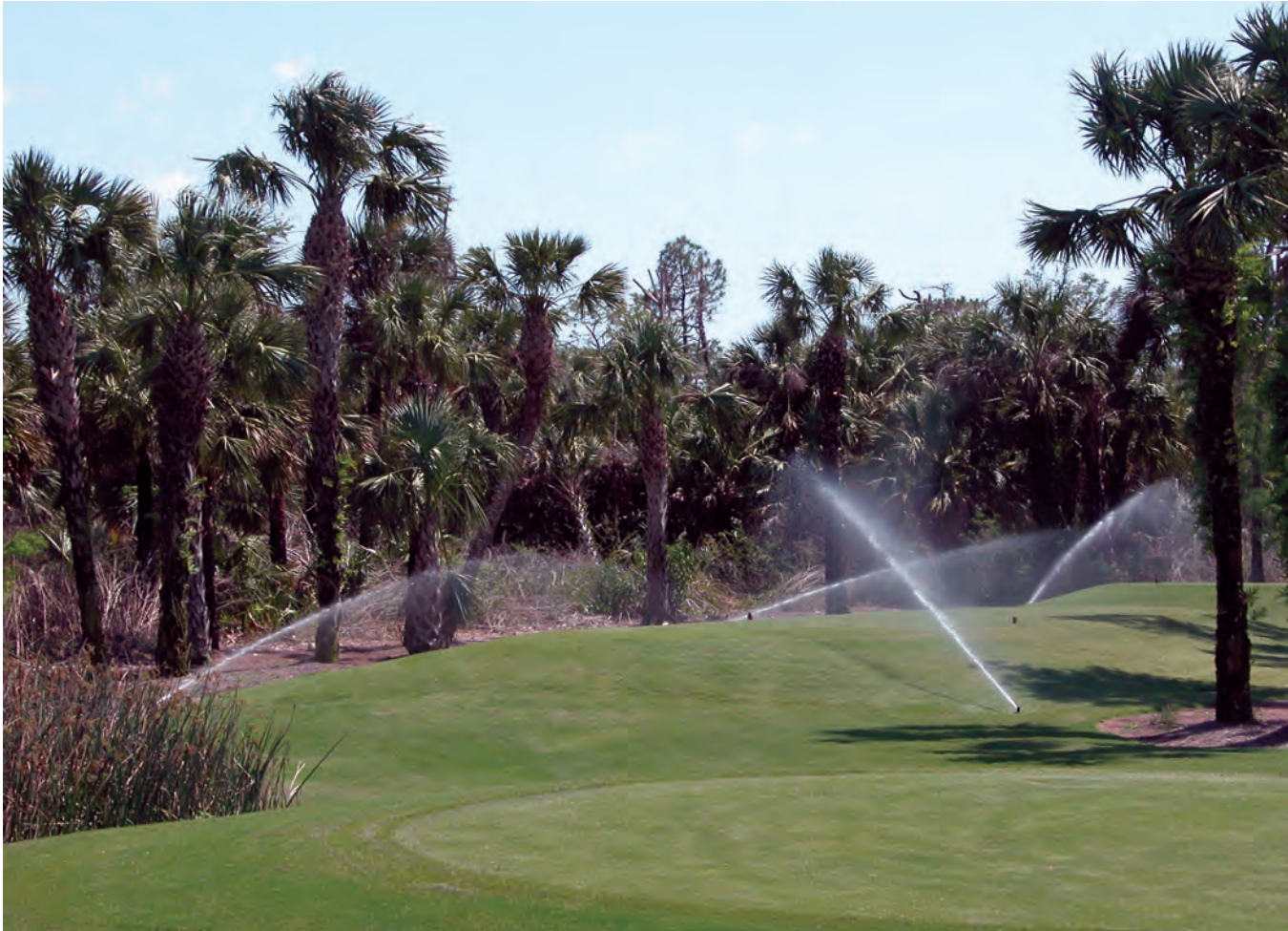
Regularly check irrigation head nozzles and operation for efficiency and conservation. Photo by Joel Jackson.
