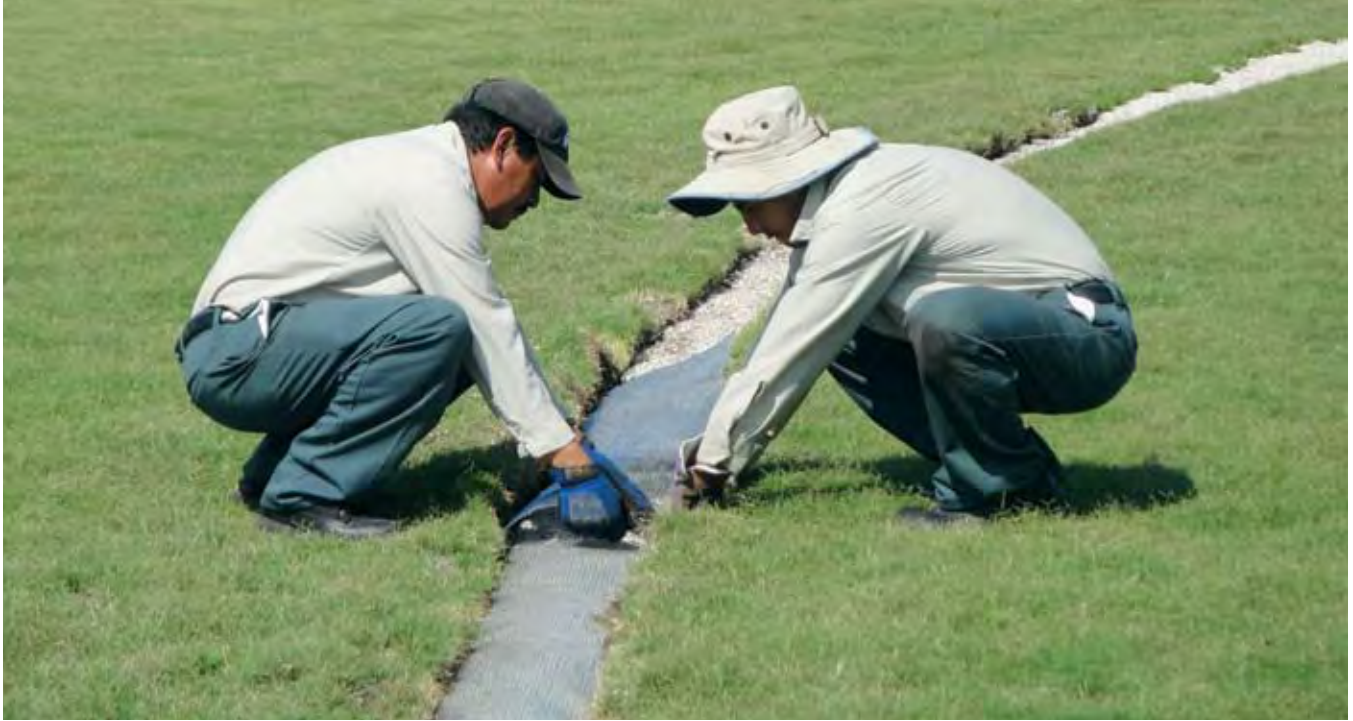
Install a strip of stucco mesh lath over the gravel layer. Photo by Darren Davis.
