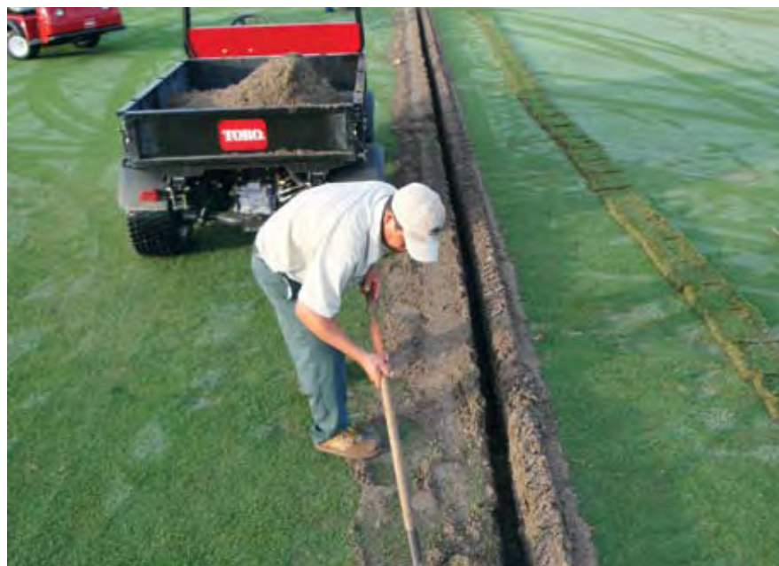
Excavate the drain line to a depth of 16 inches and 12 inches wide. Photo by Darren Davis.
