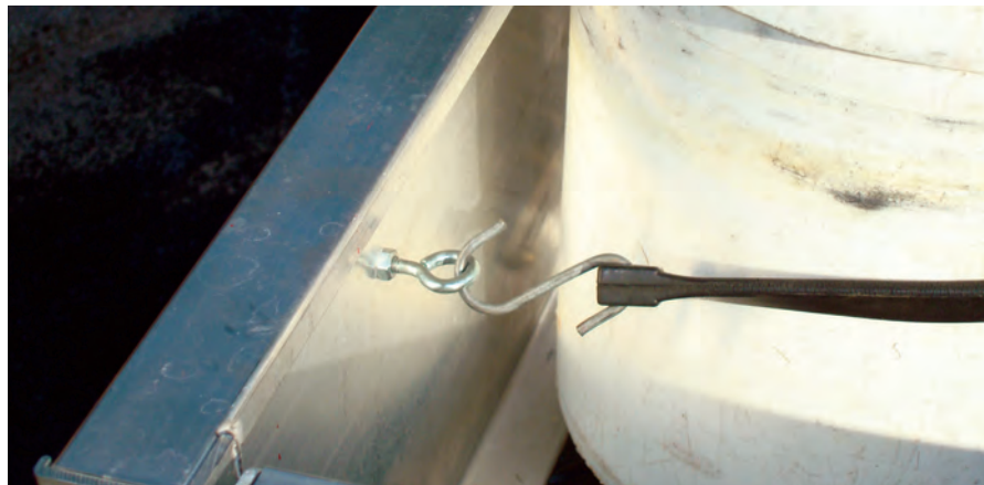
Two 1/4-inch eyebolts and a 21-inch strap with an S-hook secure the bucket. Photo by Darren Davis.
