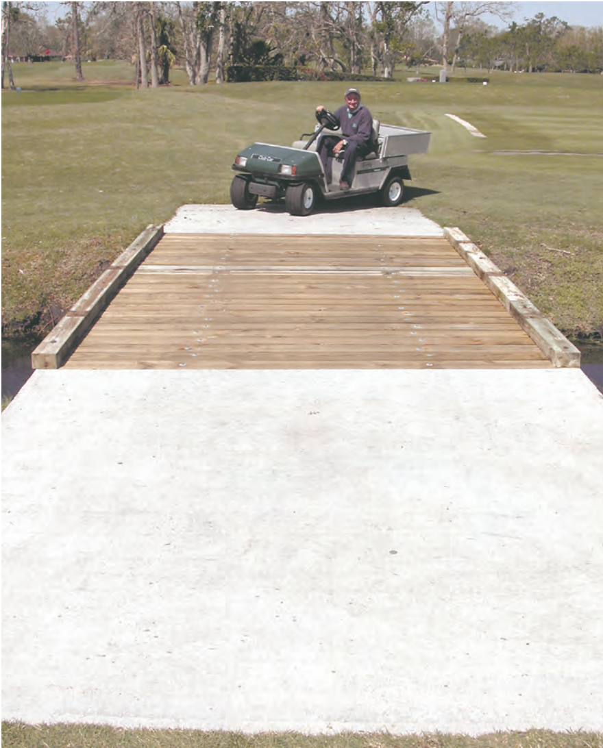
One of eight new bridges installed by the Winter Pines staff. Photo by Joel Jackson.
