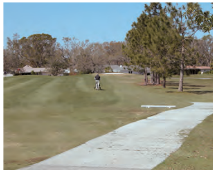
New 7-foot wide concrete paths replace and re-route the old asphalt paths. The crew often led by the owner Ed McMillin pours the new path in 110-foot long sections, which equals one truck load of concrete. Photo by Joel Jackson.
