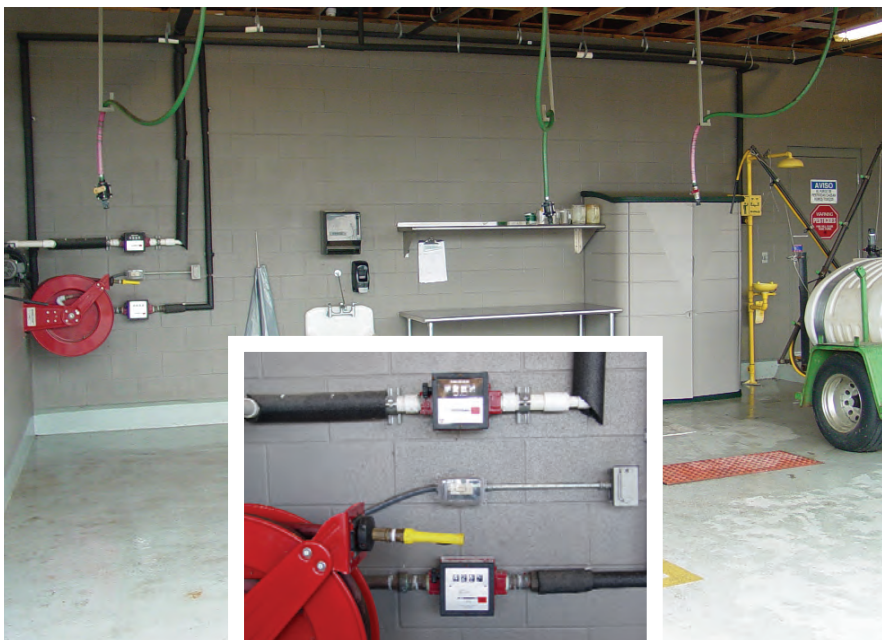
This is the main mix/load area. The concrete floor has a 36-mil chemical-resistant liner underneath and is sealed on top with chemical-resistant epoxy paint. The red grate covers the primary sump. A stainless steel mixing table, sink, eye wash and shower are some of the safety features. The recycled rinsate water is stored in a 500 gallon tank to the left. Photo by Larry Livingston, CGCS.
