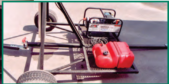
The lights are powered by a 2700-watt generator with fuel supplied by a 6-gallon marine fuel tank, both mounted on the bed of the trailer.
