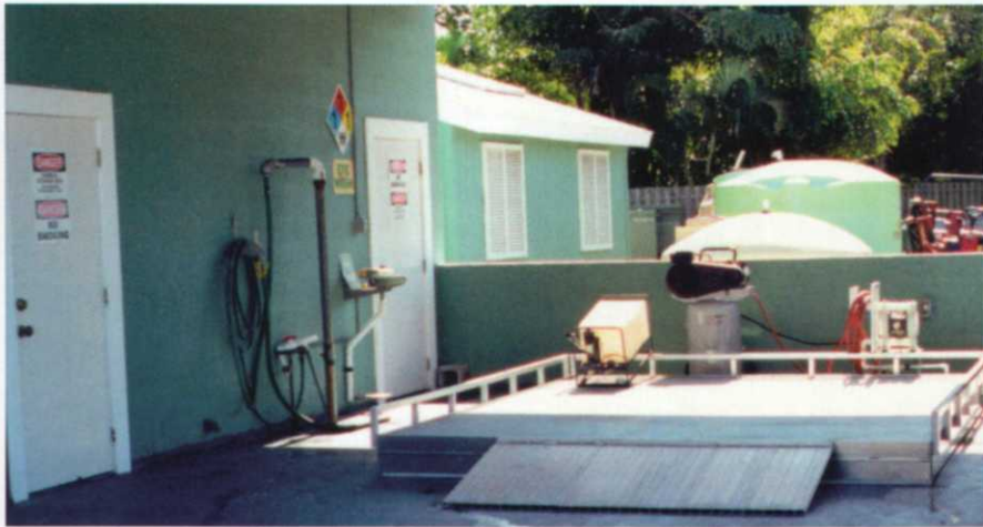
Portable 400-gallon-capacity containment skid with portable sump pump located on sealed concrete floor in protected mix-load area. Photo by Kyle Sweet.
