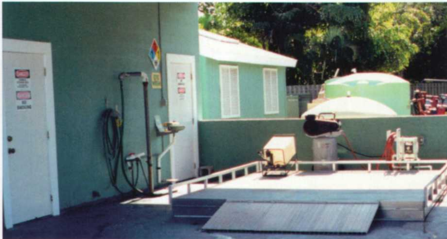
Portable 400-gallon-capacity containment skid with portable sump pump located on sealed concrete floor in protected mix-load area. Photo by Kyle Sweet.
