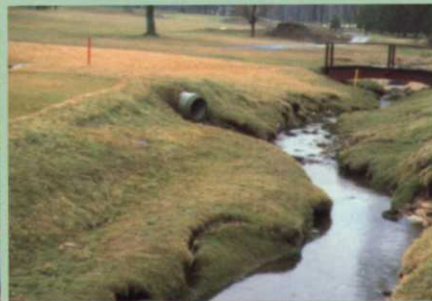
Raising the height of cut to create a turfgrass buffer zone along this creek bank at the Mendham G&T Club in New Jersey could have helped to prevent the erosion. Photo by James Baird.
