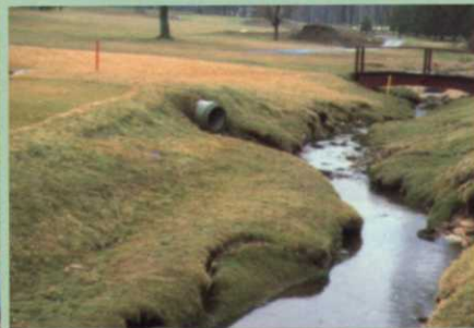
Raising the height of cut to create a turfgrass buffer zone along this creek bank at the Mendham G&T Club in New Jersey could have helped to prevent the erosion. Photo by James Baird.
