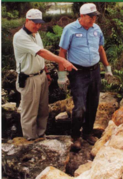
Jeff Klontz (left) inspects work progress on the waterfall project with Lloyd McCumby.
