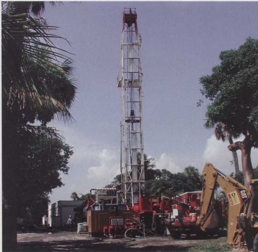
To comply with restrictions on withdrawing brackish water from the surficial aquifer during drought conditions, The Everglades Club installed a well into the deeper saline Floridan aquifer to provide water for its reverse osmosis plant to irrigate the golf course.
