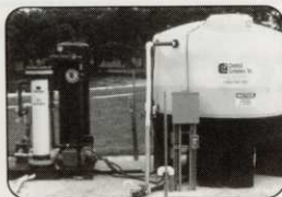
Wash Rack Systems – •closed loop •sewer discharge
