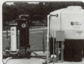
Sewer Discharge System
