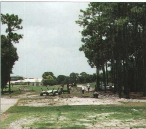
Irrigation contractor at work installing a new system on the South Course. Mike has his plate full with three or four projects underway this summer!
