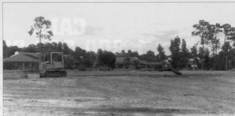
Big noise — The roar, thump and clank of heavy construction equipment has been a summer-long constant on The Forest's rebuilt Bobcat course. Looking back toward the tee, the fairway on No. 16 has been recontoured, its drainage improved. Photo by Bill Kilpatrick.
