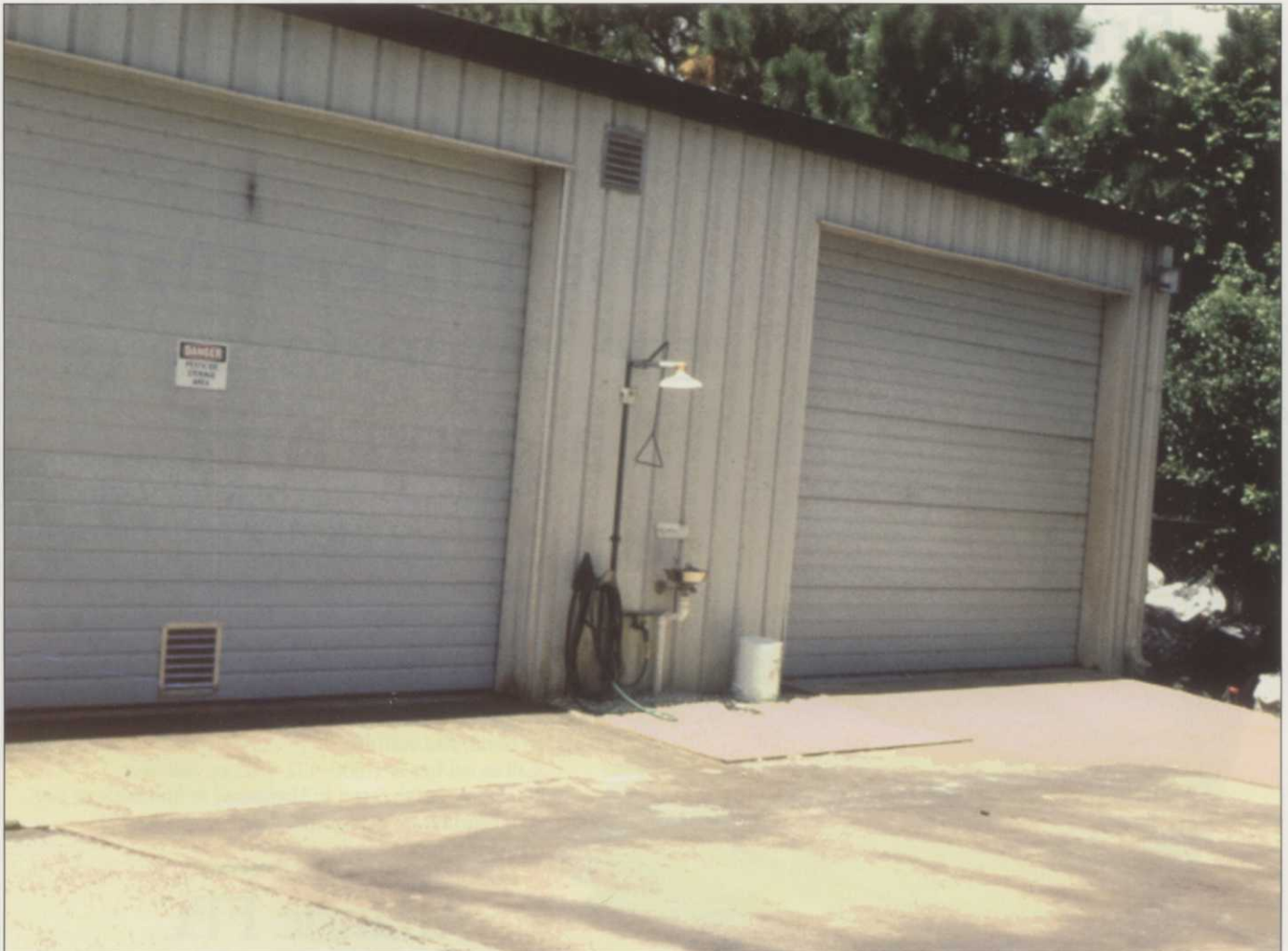
Emergency eyewash and shower station at the chemical room is not only common sense but a well founded regulation.
