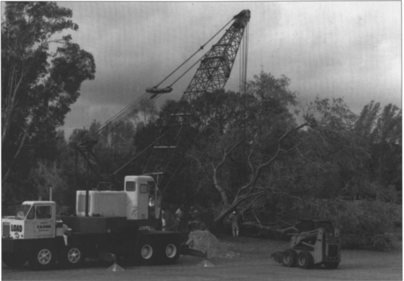
A 40-ton crane is used to lift a fallen oak tree at Don Shula's Hotel and Golf Club, Miami Lakes.
