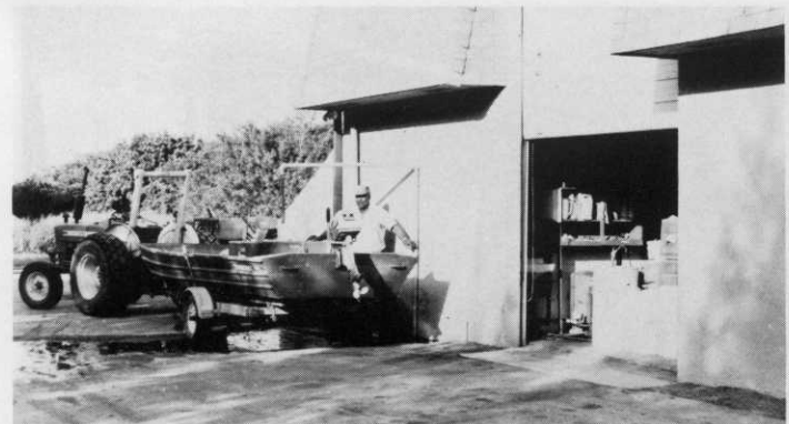
Boca Greens chemical room is designed with easy entry, concave floor with drain, sink, and outside hose bib. ■
