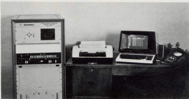
MIR-2100 CENTRAL STATION, City of Los Angeles Encino Golf Course (Installed by California Engineering, Sylmoor, CA)
