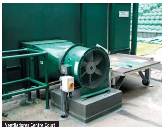
Ventiladores Centre Court
