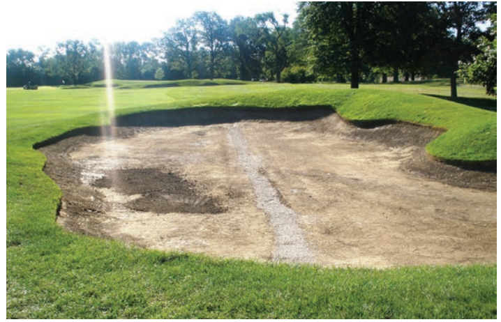
The bunker project began: Members had lots of ideas on what they'd like to see done, but we had to be practical.
