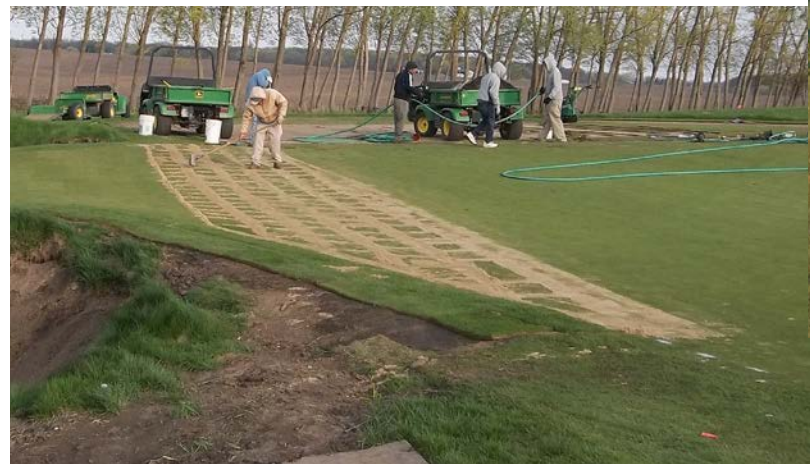
Black Sheep staff topdressing seams on new sod and preparing new bunkers for liner installation during the early spring of the year.
