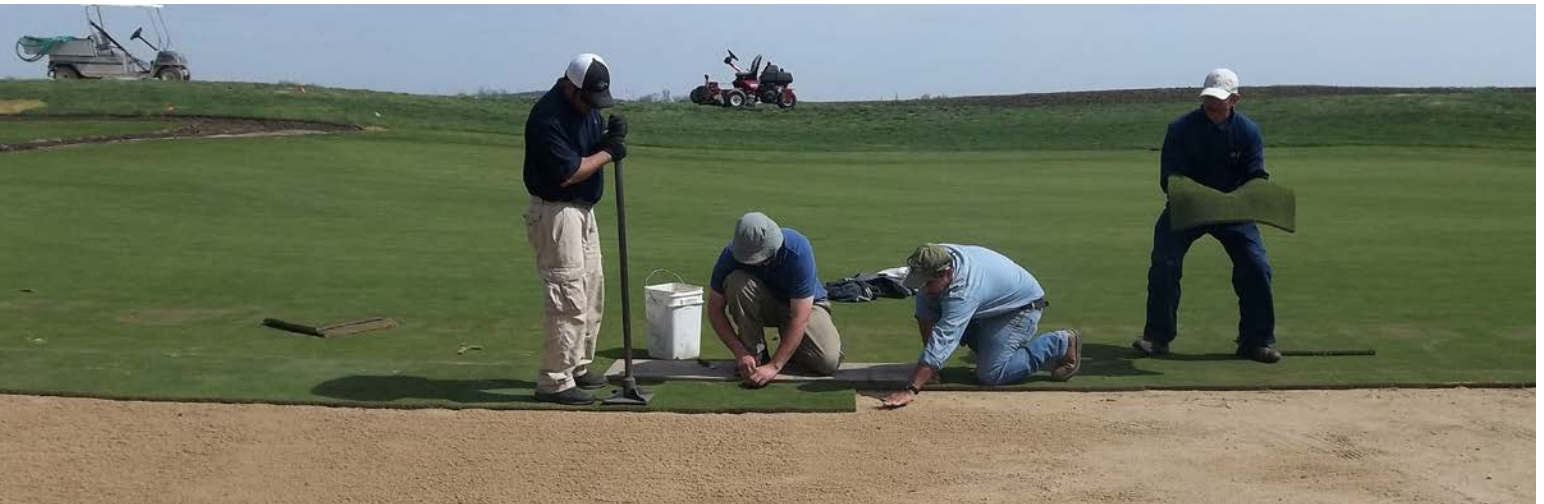
Staff carefully moves sod from existing section of the green to the new portion. Green was constructed using the California method of putting green construction.
