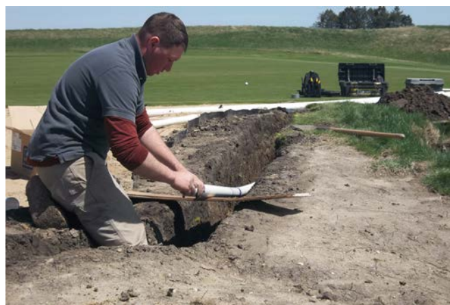
After measuring proper irrigation head spacing, the staff re-routes lines and places piping for each head.
