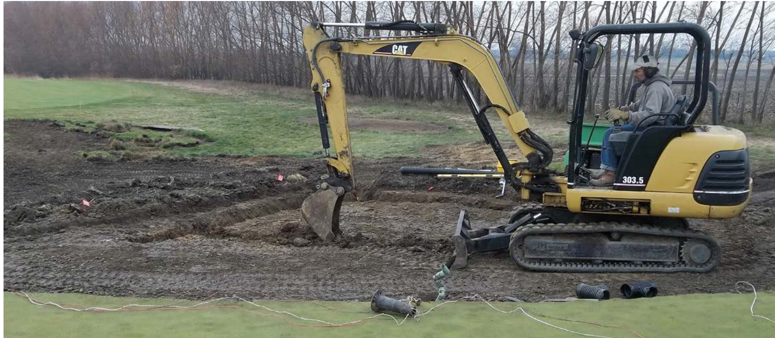
Mike Reardon begins to cut drainage trenches to tie the new part of the green into the existing drain lines.
