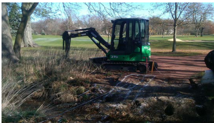
IHC rented a mini excavator to dig footers and properly place the pipes within the ditch.
