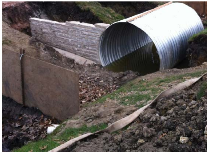
The plywood in the forefront was used to temporarily damn the water. As the water rose, pumps were used to transfer water to the low side of the ditch.
