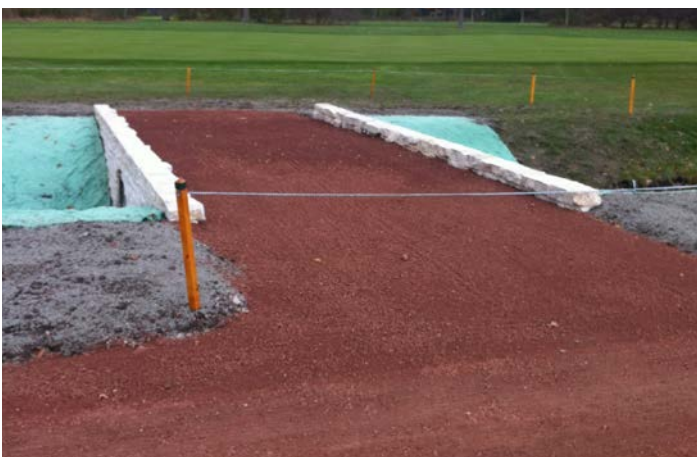
After each bridge complete and backfilled, staff finished off the grade with crushed red stone to match the existing path work at IHC.
