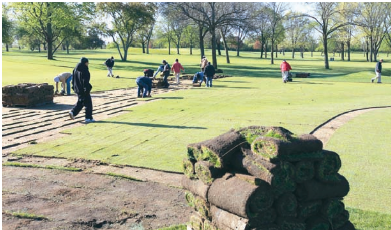
The clock starts ticking. The crew takes advantage of the dry spring to strip a low area in a fairway. The ground will be re-contoured to increase surface drainage and the sod replaced within a few days before the sod expires.
