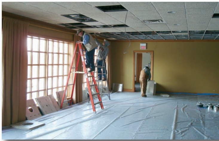
Members of the grounds staff install new drop ceilings in the dining rooms this winter. It saved on the cost of the project and allowed Tim to keep staff members throughout the winter months.
