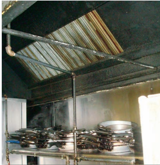
Instead of outsourcing all of the maintenance in the clubhouse, staff is used to clean exhaust baffles in the kitchen.
