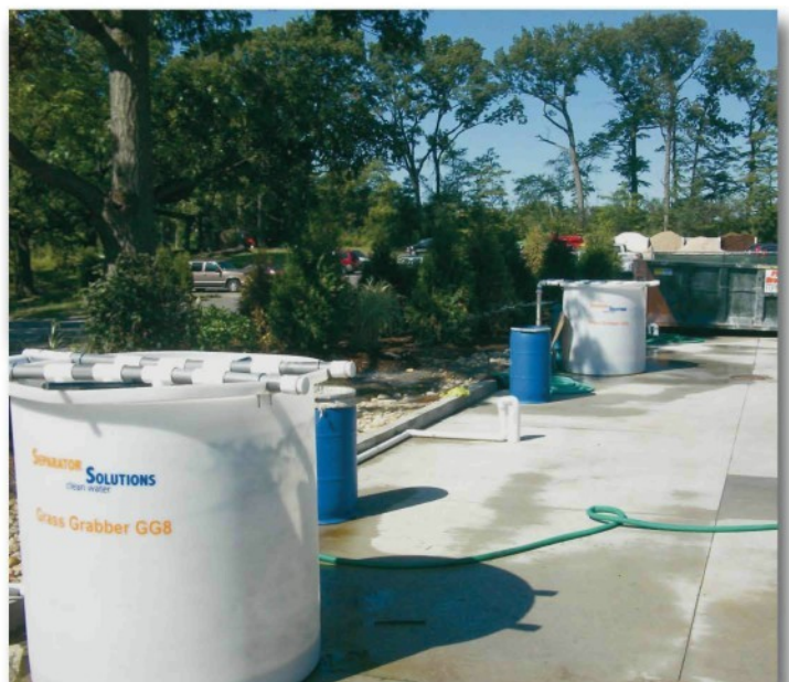
The wash pads drum and basin system at Medinah Country Club. (continued on next page)
