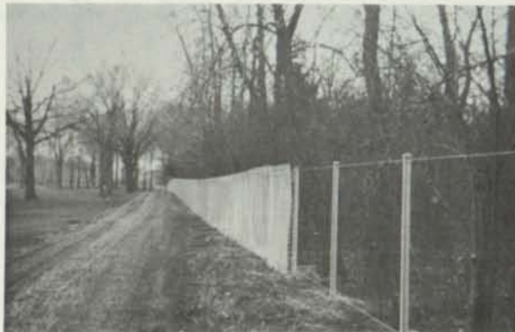
Cyclone fence being installed at Bob-O'Link Golf Club. Part of a 3-year program.
