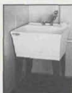
Wash tub with emergency eye-wash
