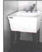
Wash tub with emergency eye-wash
