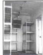
Propane or natural gas heater.
