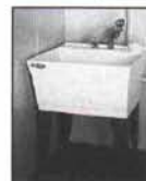
Wash tub with emergency eye-wash
