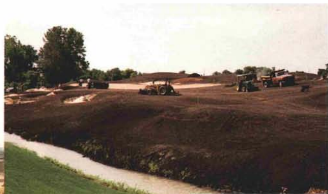
8/5/92—Activity abounds during all phases of construction, especially finish grading and seedbed preparations.
