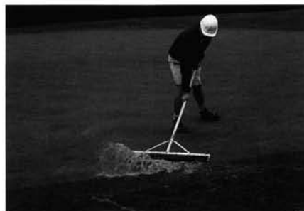
Standing water on greens that requires squeegeeing following heavy rainfall is an obvious sign of poor surface drainage.
