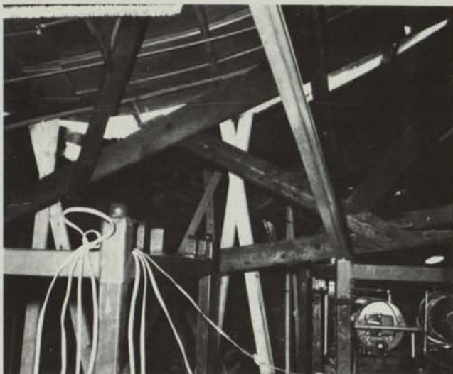
Snow damage to roof at Ill. Lawn.
