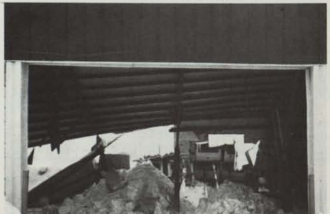
Equipment building after the roof collapsed, due to heavy snow at Silver Lake C.C.
