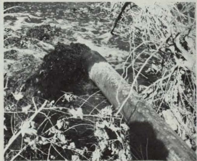
The November issue of the BULL SHEET showed a picture of a dredge or mud-cat working in Gerber's pond at Glen Oak C.C. The above picture 1/3 mile away shows where the mud from the bottom of the pond is being discharged. A neat operation. A good way to clean out the old lake.
