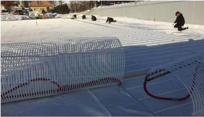
A pipe grid is customized to the shape of the rink and can keep ice around from November to March in the Chicago area.
