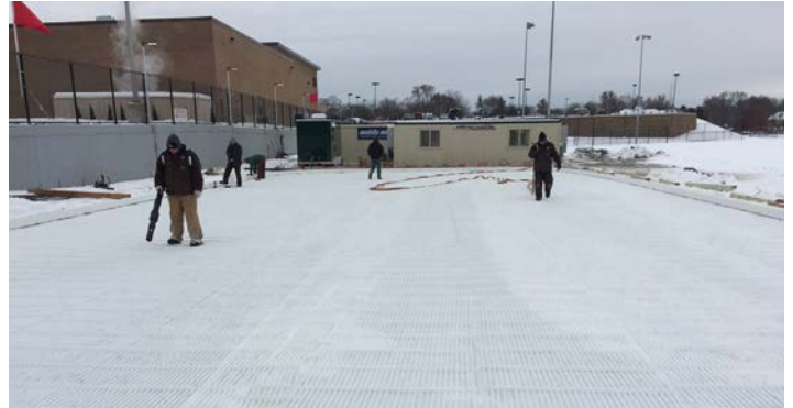
Wheaton Park District and owner of Arrowhead Golf Course recently installed a new ice rink system using the same chiller they use during the summer months to air condition their fitness center. Page 8.
