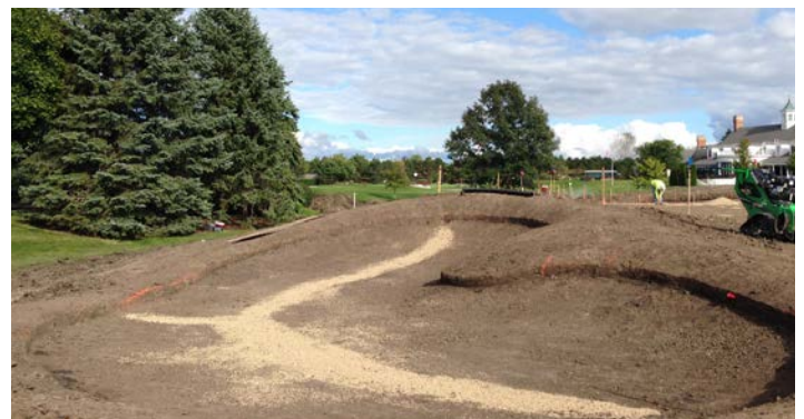
Flashed-sand construction is a valid option again in wetter climates without the worry of erosion and contamination.
