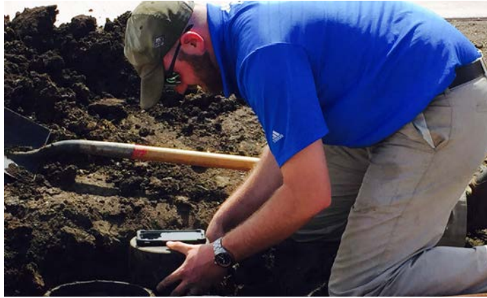
Andrew Cross at Arrowhead comes up with another use for his phone, making sure sprinkler heads are level using the phone's built in accelerometer and a level app.
