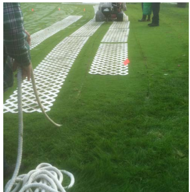
A vibratory plow is used to install the drainage element into the soil with minimal disruption to the surface.
