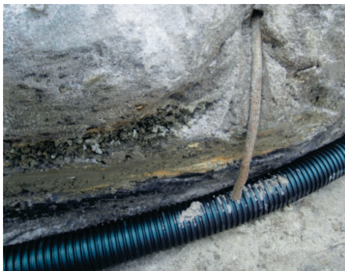
The discharge end of the PC Drainage is hooked up into existing or new conventional drain lines.
