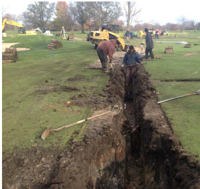
All the soil was removed from each trench cut on the property and backfilled with sand.
