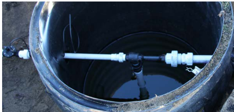
One of the Irrigation Drive Pumps (IDPs) in the early stages of installation in a sump. They sound more complicated than they really are.
