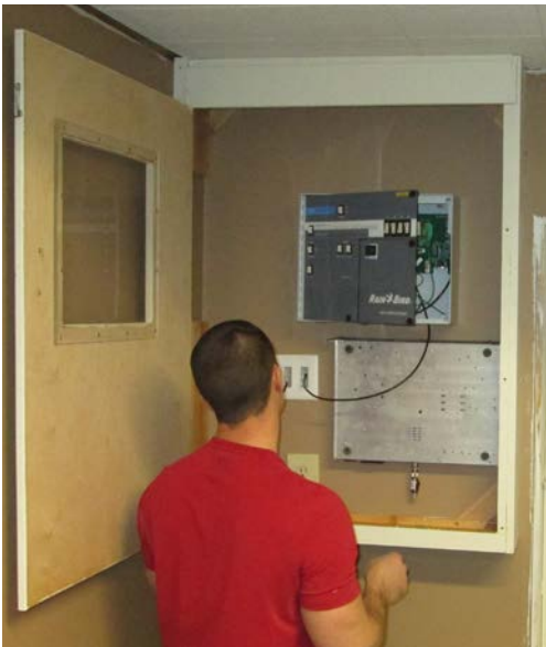
Jason re-installed the irrigation controls into a custom built housing that will neatly hide all the wiring.
