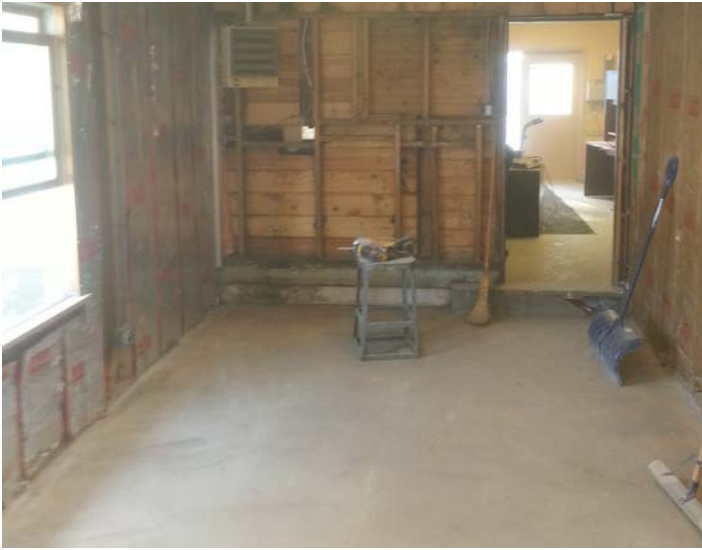
Removing wall paper is easiest when you take out the wall board that it is glued to.
