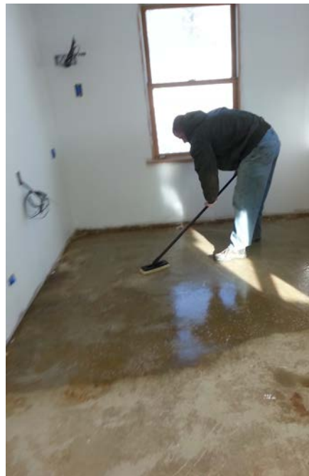
Etching the bare concrete floor ensures that it is clean and good adhesion for paint.
