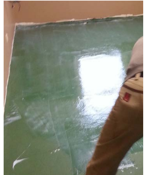
Dan added a coat of concrete semi-gloss to the floor to keep it shiny and easy to clean.
