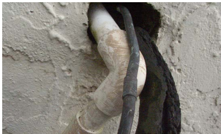
A lot of energy is lost where pipes run through exterior walls. Cans of expanding foam are a simple, inexpensive fix.
