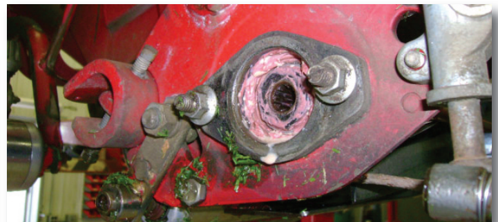
Above: Grease and water don't mix.
